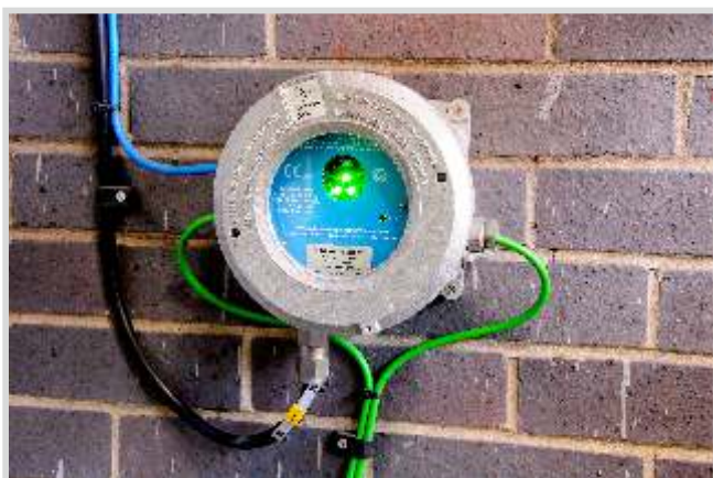
Figure 2: Traditional wall mounted ground status indicator system with internal output contacts. Note the green for 'SAFE TO GO' indication method.
