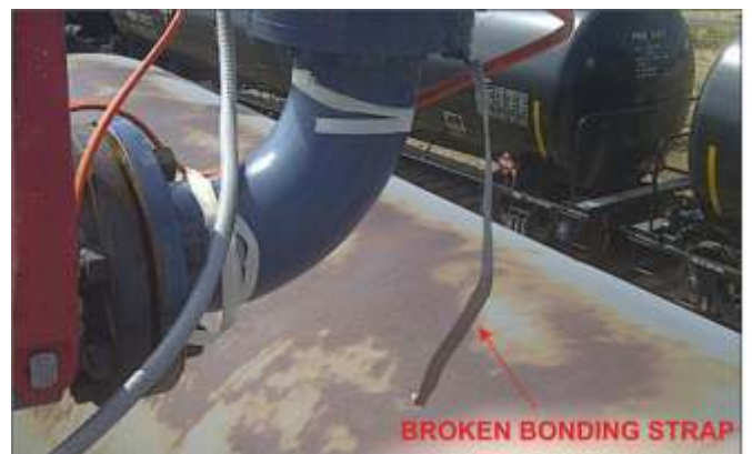
Figure 3: regular audits of a site can highlight safety risks similar to the broken bonding strap highlighted above.
