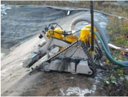
Fig 1: WEDA robot equipped with electric cable, for operation of the pump, and 75 mm hose, for the transportation of sludge to Geotube.
