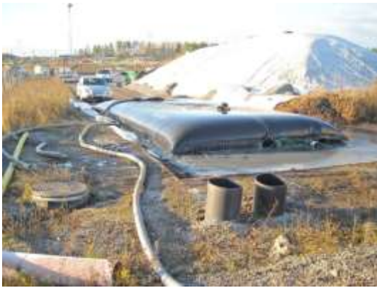
Fig 2: Geotube after about eight hours filling of sediment, sludge about 1-6% DM, pumped with WEDA-robot. DM content in Geotube increased to > 20%. NOTE: The addition of flocculating chemicals about 5 meters before the entrance to Geotube.
