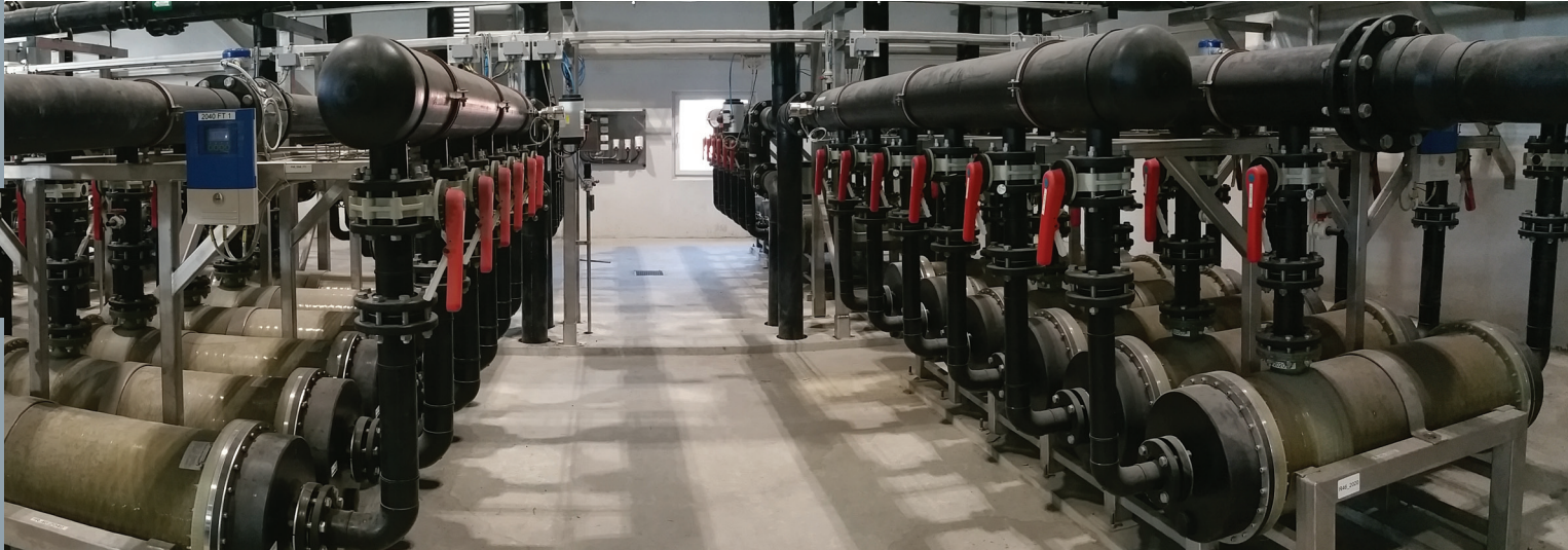
Metal transformation plant SWEDEN
