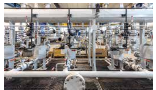
Condensate lift station
