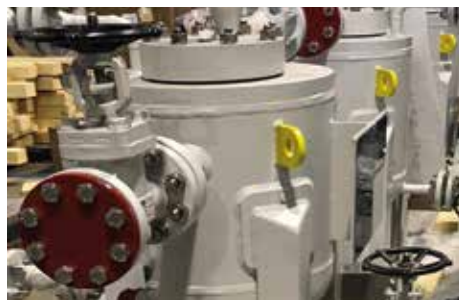
Condensate lift pump
