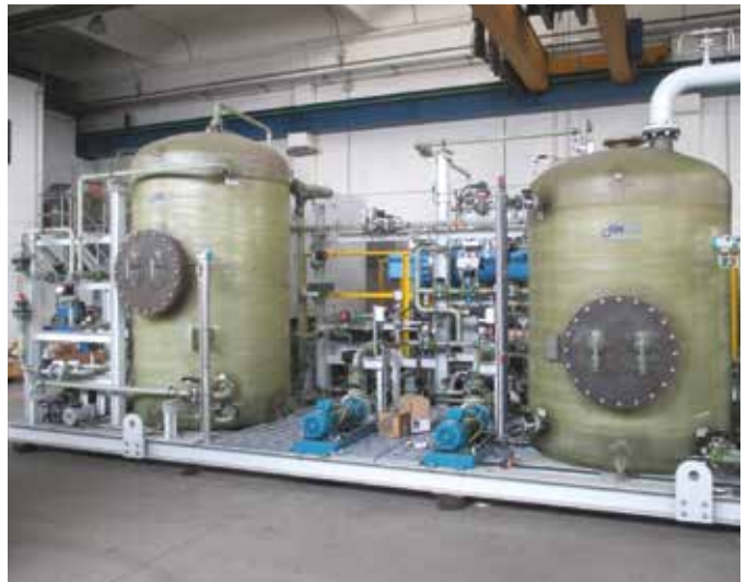
Electro Chlorination System
