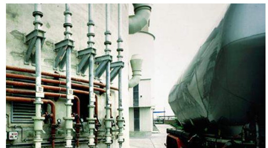
SILO FILLING WITH PINCH VALVES
